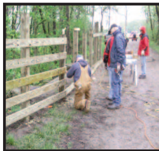
Twenty volunteers worked through a light rain setting through a light rain setting posts and installing railings at both Rattlesnake and Tank Car Culvert to fully complete this section of trail.
