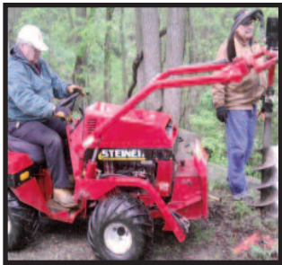
Long time FRTTI Volunteer Stan Bernhardt laid out the bridge railing plans at Rattlesnake Creek and the culvert near Rt 601. Rich Libbee drilled a lot of holes in advance.
