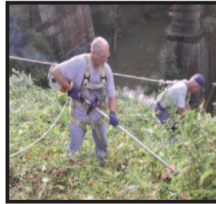
The Norwalk Double Arch Bridge got a trimming this fall as Steve Siesel and Doug Jaqua clear the top. Drainage work will take place this summer.
